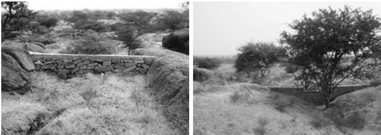
Fig 3.10. Loose stone check dam (left) and masonry check dam (right) for treating drainage line.
