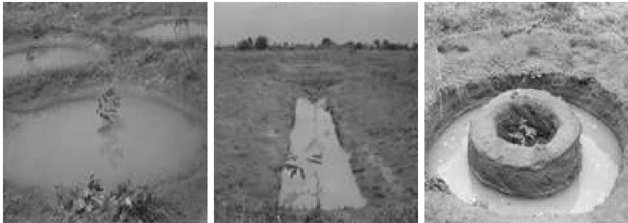
Fig 3.4. Different micro-catchment rain water harvesting structures like saucers pit (left), ridge and furrow structure (centre) and ring pit (right).
