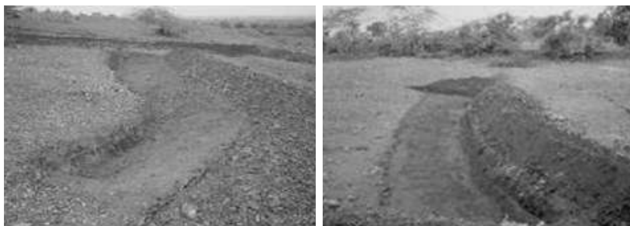
Fig 3.8. Gradonies (left) and V-ditch (right) rainwater harvesting structures under rehabilitation of degraded lands. Source: Singh (2011).
