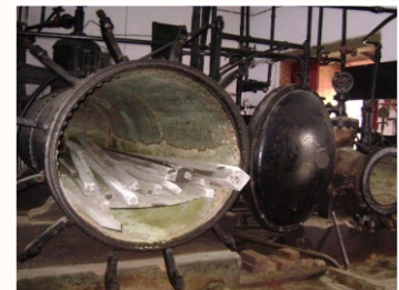
Pressure Treatment Plant
